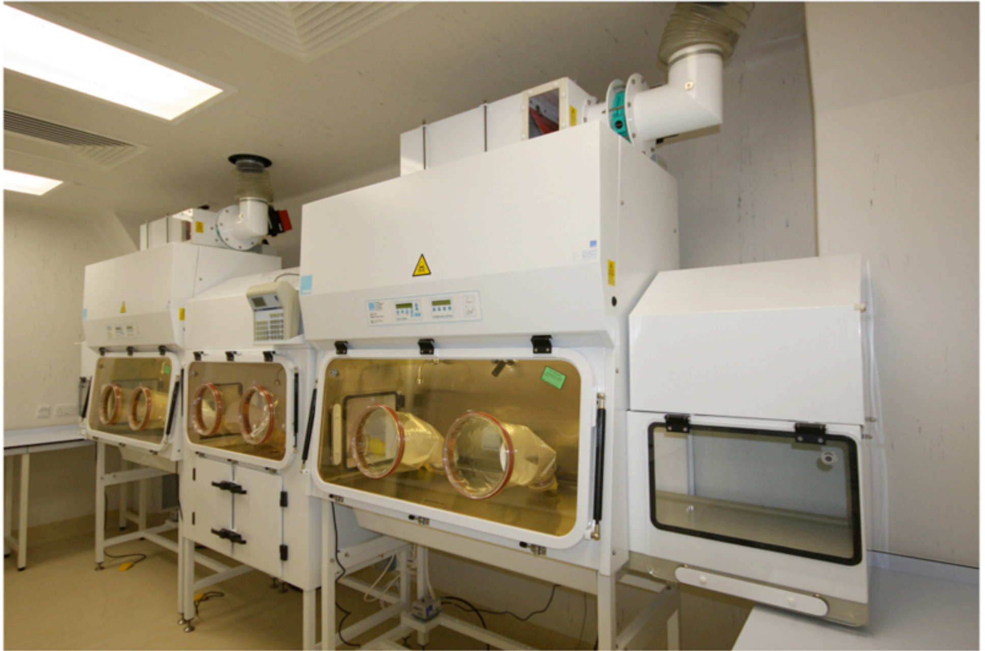
Dual chamber transfer from Tc generator
